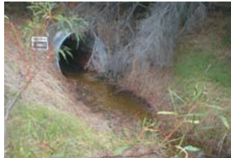
Despite south-west WA experiencing the driest year on record, recent high tides have resulted in rising groundwater inland from Mangles Bay. Photo – Hugo de Boorder
